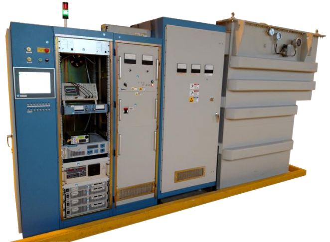
Fig. 1. ESS Klystron Test Stand, showing controls and auxiliary supplies in the left cabinet, the high voltage power supply (center-left), the high voltage modulator cabinets (center-right), and transformer (far right).
