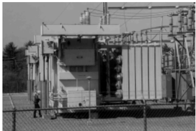
Figure 2: 115kV to 13.8kV AC Transformer
