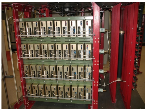
Figure 3. Switch plate array in the transmitter's modulator. The entire assembly is submerged in oil.
