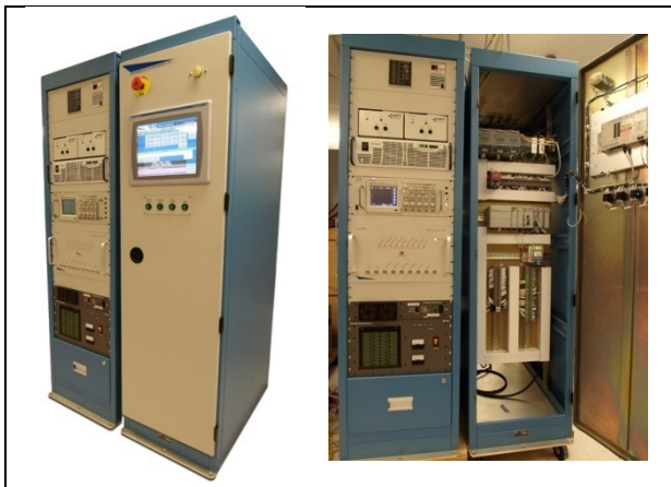
Figure 6. Controls racks for the 2 MW klystron transmitter.
