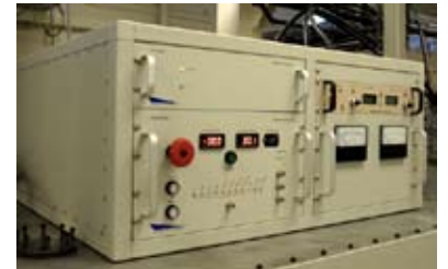
The test stand's modulator controls include fast fault detection and first fault identification.
