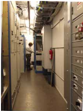
Shelter interior showing typical arrangement of transmitter components. DTI recently delivered X-band and S-band solid state, transportable radar transmitters configured in standard 45 foot, weatherproof ISO shelters to the U.S. Government.
